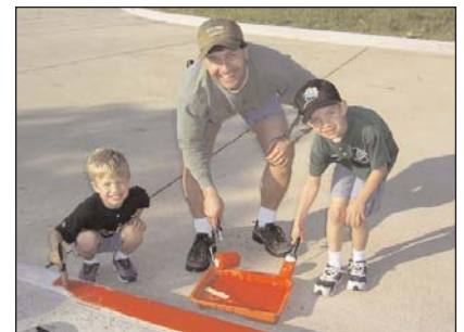
A family from Fellowship Bible Church North works together striping the parking lot at the museum renovation project.
